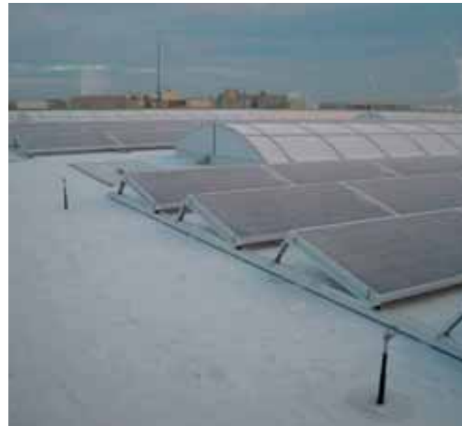
Installation of photovoltaic panels on the warehouses at DP World Breakbulk in Antwerp, financed by Dexia as part of its Dexia Energy Line – Renewable Energy offering
